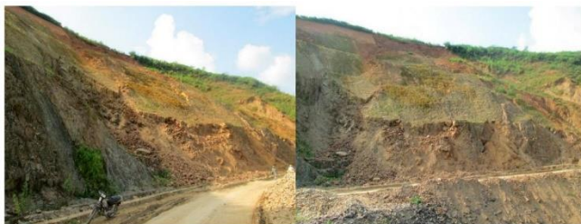
Figure 2. Two photos of the landslide on the slope wall of National Road 279, near the right bank of Nam Kim stream, Na Pa village, Muong Kim commune, Than Uyen district. Source: Vietnam Institute of Geosciences and Mineral Resources [29]
